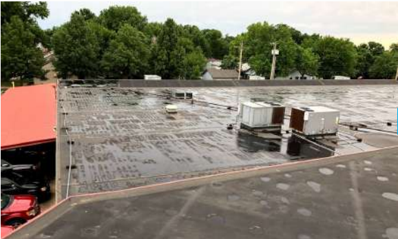
Roof at end of life
