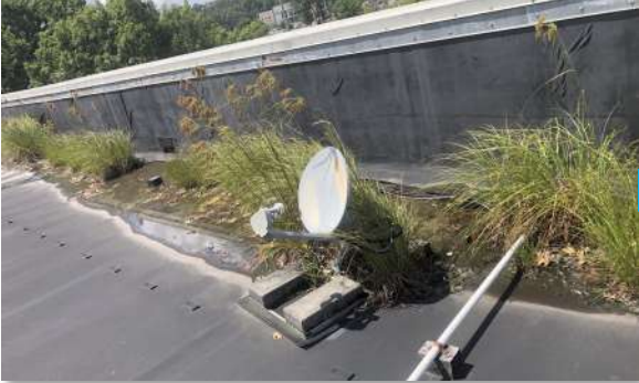
Dirt and debris buildup
