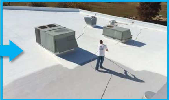
Entire roof receives a minimum of two full coats of ASTEC Finish
