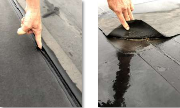
Failing seams and mastics
