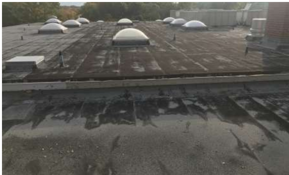
Roof at end of life
