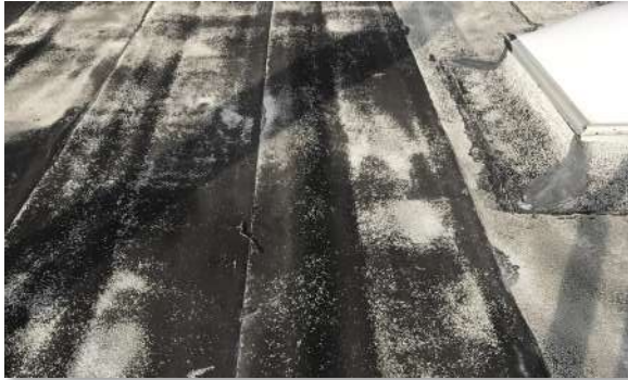
Ageing membrane and loose granules
