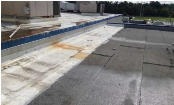
Failed coating products
