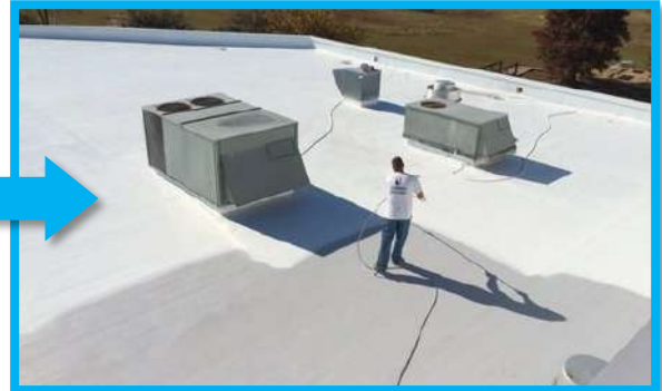
Entire roof receives a minimum of two full coats of ASTEC Finish
