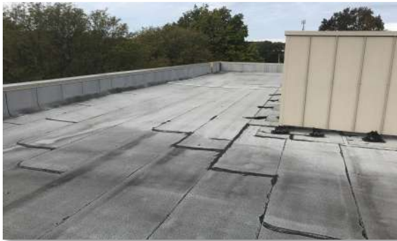
Failing seams and mastics
